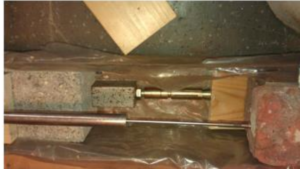
Figure 11.6: Between the stones and the wooden plank a spanner is placed to prevent sliding of the plank
